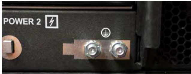
Figure 6: Chassis ground lug
