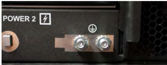
Figure 6: Chassis ground lug
