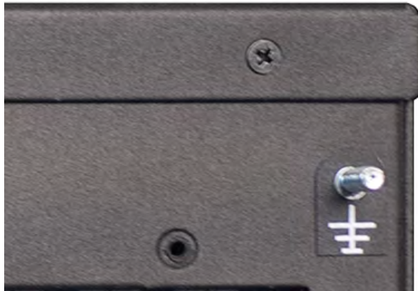
Figure 6: Chassis ground lug
